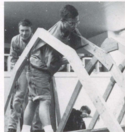
Justin, Ian, and Jeremiah work hard to complete this storage shed by spring. Looks good so far!
